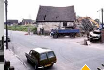
The demolition of the water mill on June 30 1975. The small brick building in the foreground was a public gents toilet. The Ropery and its manager's house are on the left. Chemical Road (now Malkiln Road) is on the right
