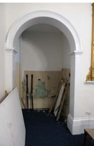
Damp in the exhibition room
